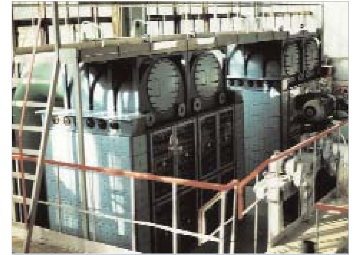
Figure 22. UV drinking water plant 405.000 m 3 per day, Tollyaytti (Russia).
